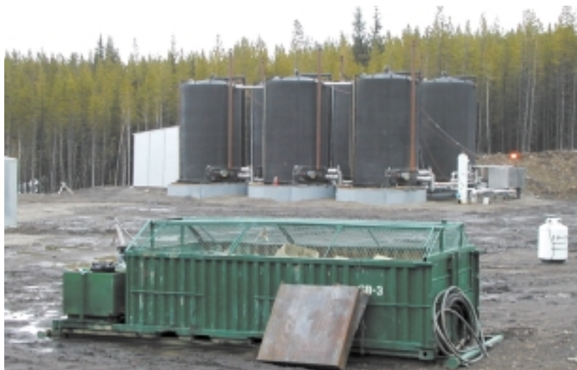
▲ Water extracted from coal seams can contain salts and heavy metals. The B.C. Government has established new standards prohibiting the surface discharge of produced water.
